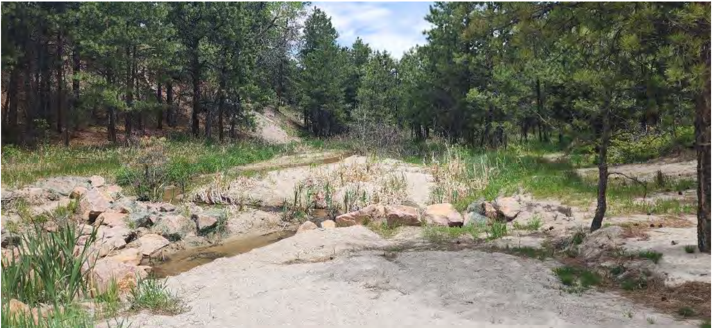
Photo Point 9 – View northeast (upstream) of wetlands and boulder grade control structure (historic open water pond) on Kettle Creek and adjacent ponderosa pine forest. Drainage 3 drops sediment in this location.
