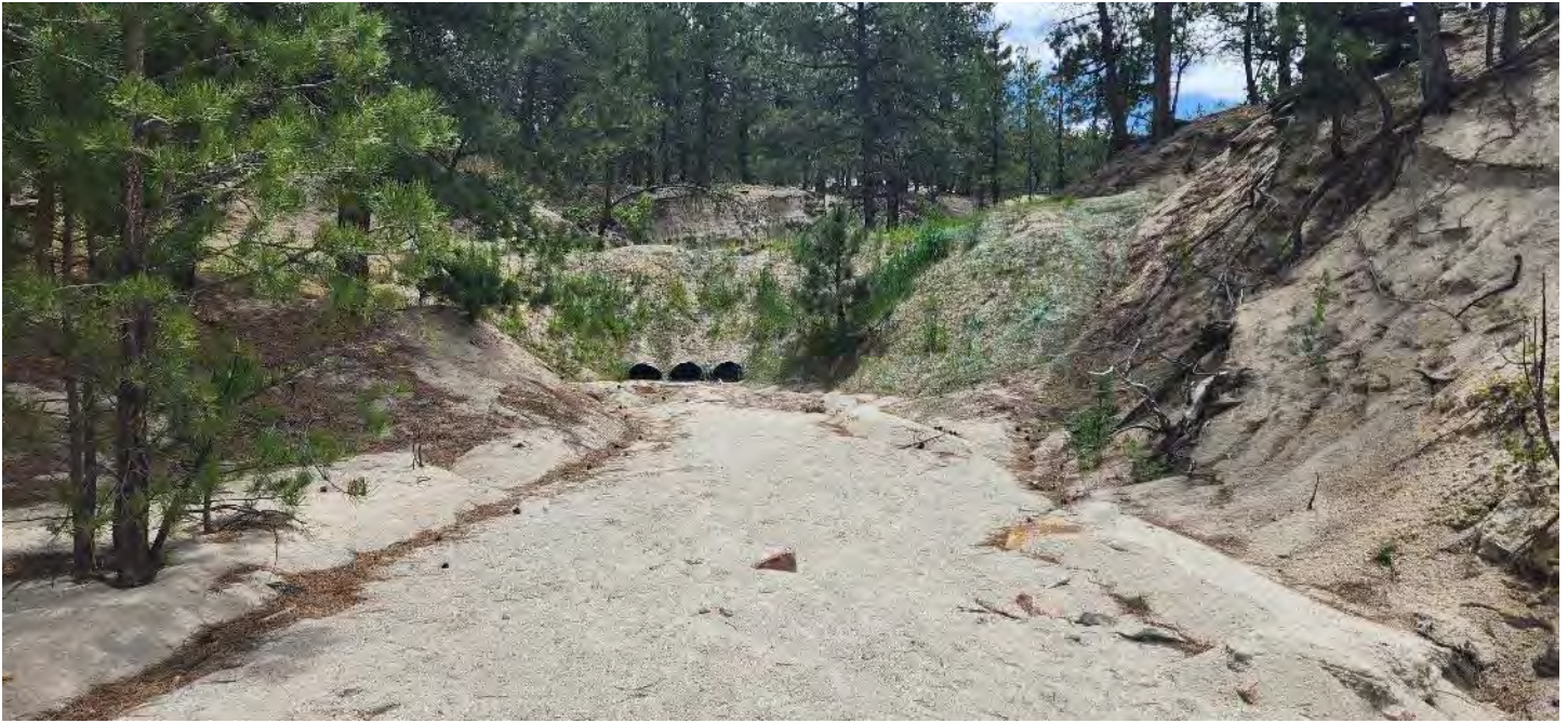
Photo Point 9 – View southeast (upstream) of Drainage 3 near confluence with Kettle Creek.
