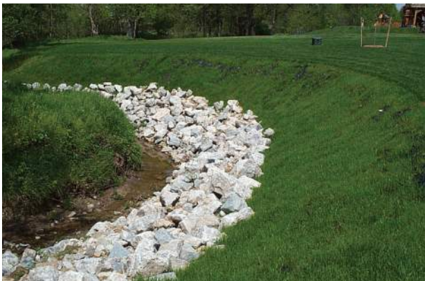
The TRMs easily conform to various landscape features to prevent the loss of precious topsoil.
