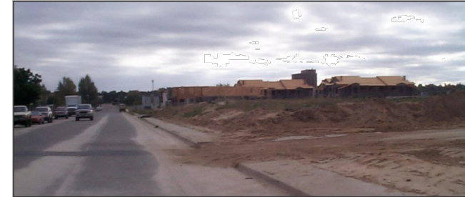
This picture shows an unstabilized entrance where dirt is being tracked onto a public road.
