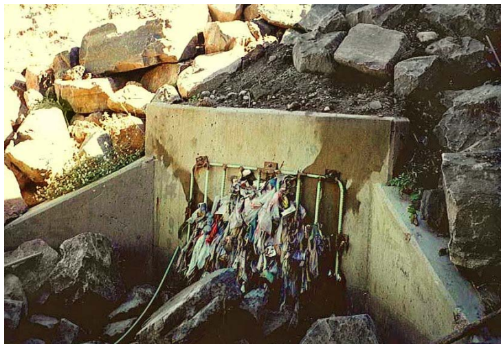
Photograph SSC-1. Storm drain cleaning may help to remove pollutant sources and helps to maintain the capacity of the storm pipes.
