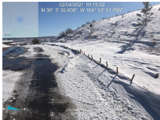
Perimeter control measures implemented along Forest Lakes Drive entrance where MVEA /waterline disturbance occurred.
