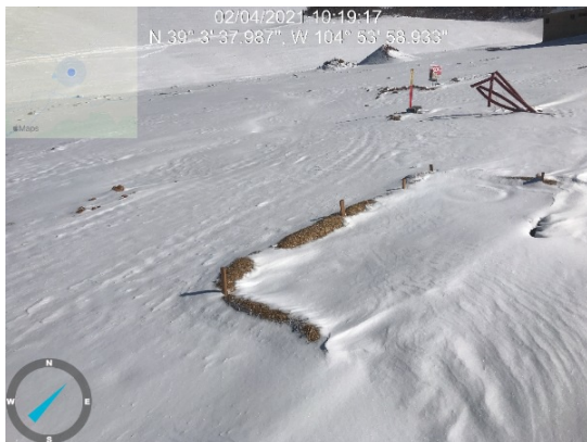
Unable to fully inspect curb inlet protections along Mesa Top Drive in F5 due to snow cover.
