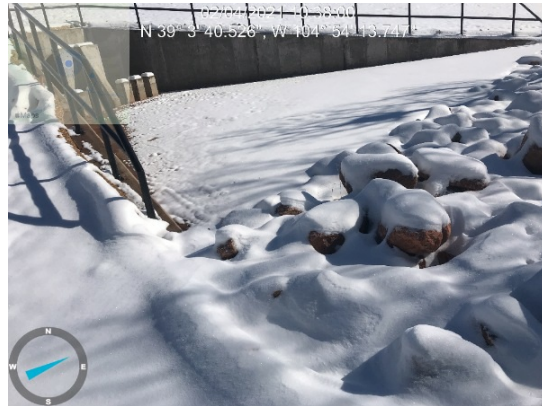
Outlet structure at end of F5 unable to be inspected due to snow cover.
