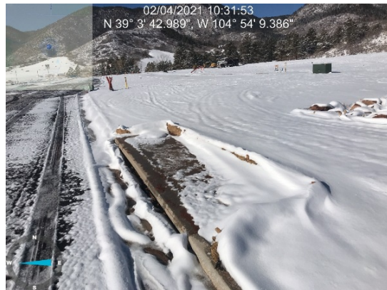
Unable to fully inspect curb inlet protections along Mesa Top Drive in F5 due to snow cover.
