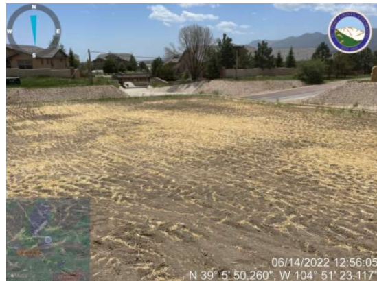
Disturbed areas have been temporarily stabilized and seeded. Straw wattle perimeter control measures remain in place.
