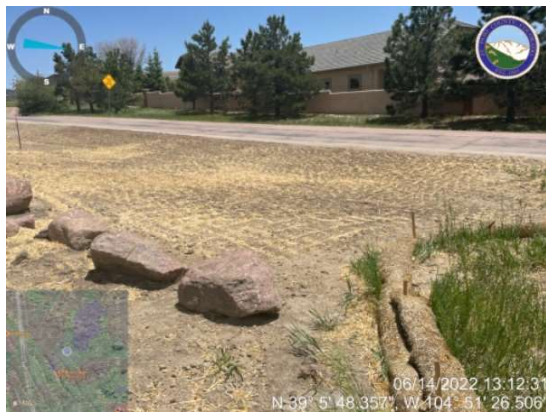
Disturbed areas have been temporarily stabilized and seeded. Straw wattle perimeter control measures remain in place.
