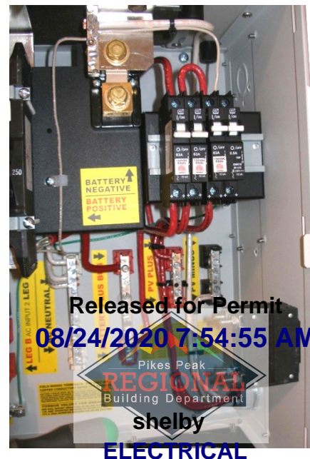
63 amp din rail DC-GFP wired with a 63 amp PV disconnect and a 63 amp controller output breaker.
