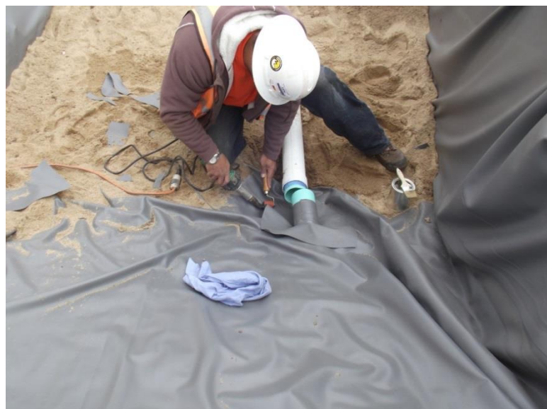
Photograph B-3. Ensure a water-tight connection where the underdrain penetrated the liner. The heat-welded “boot” shown here is an alternative to the clamped detail shown in Figure B-2.
