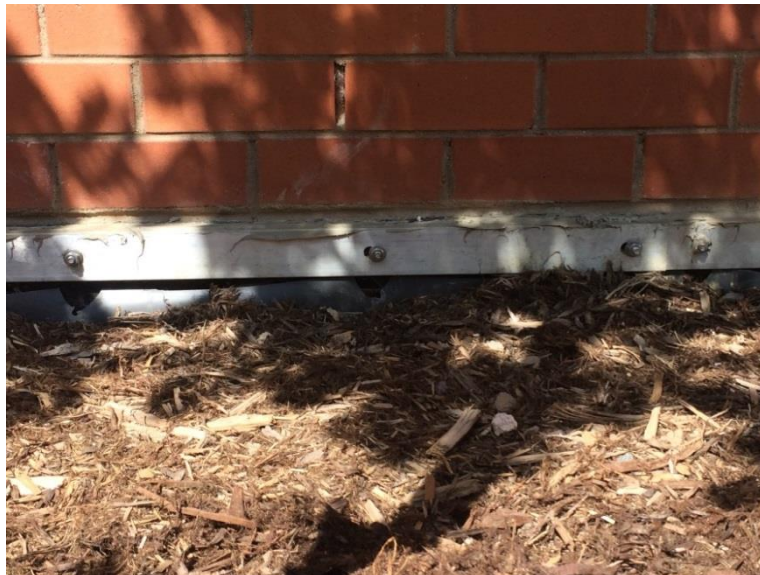
Photograph B-2. The impermeable membrane in this photo has ripped from the bolts due to placement of the media without enough slack in the membrane.
