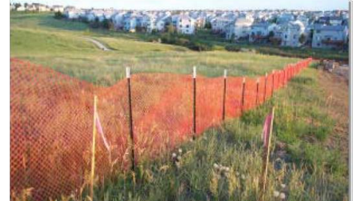
Photograph CF-1. A construction fence helps delineate areas where existing vegetation is being protected. Photo courtesy of Douglas County.
