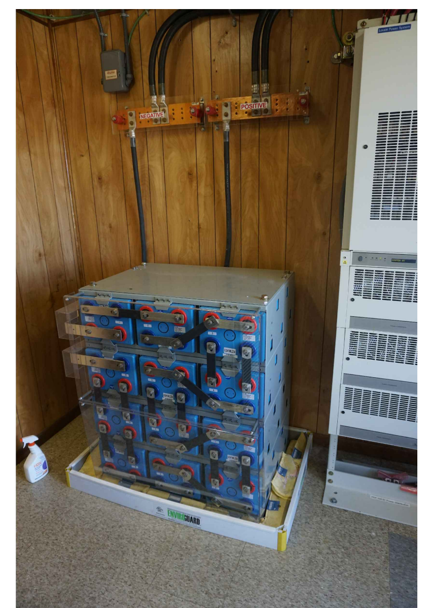
INTERIOR VIEW: BATTERIES
