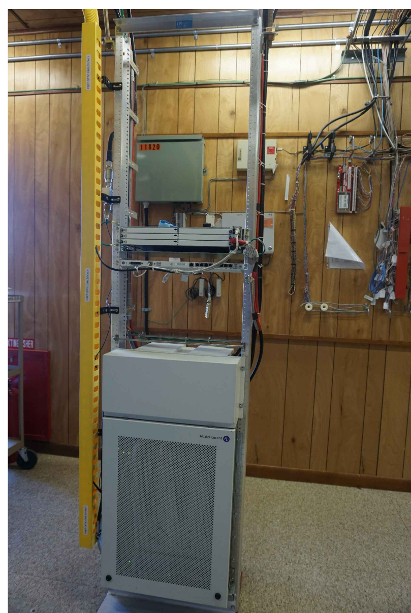
INTERIOR VIEW: E-NODE B/BBU RACK
