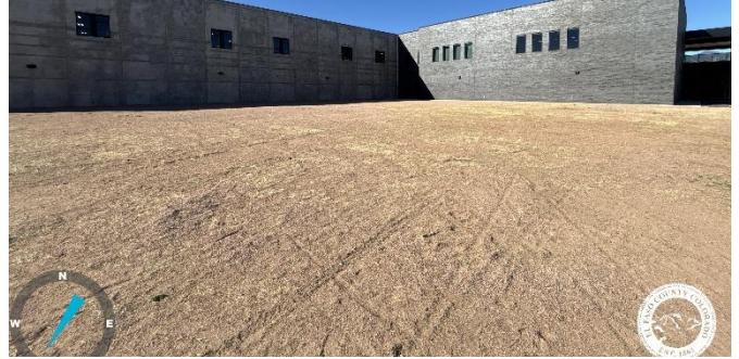
Photo 14: Northeast of building. Vegetation has not met requirements. Update Pond Calcs and As Builts to show this impervious area or stabilize.
