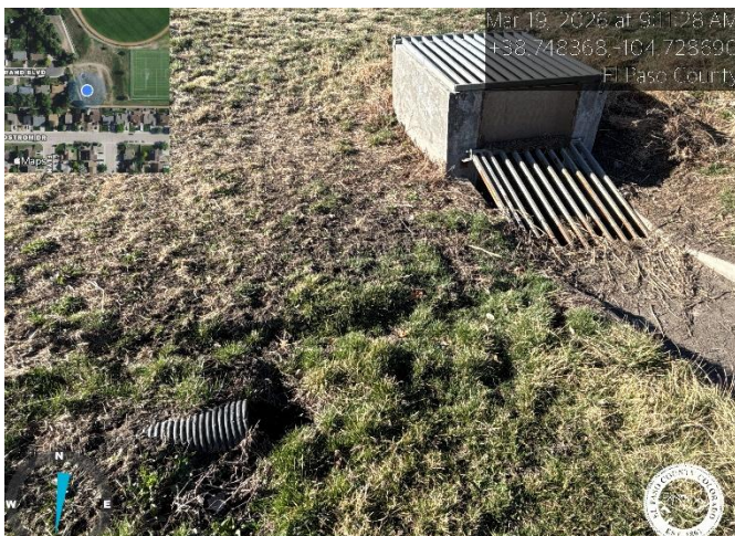
Photo 7: Inlet pipe in pond bottom not shown on plan. Show on as-builts.
