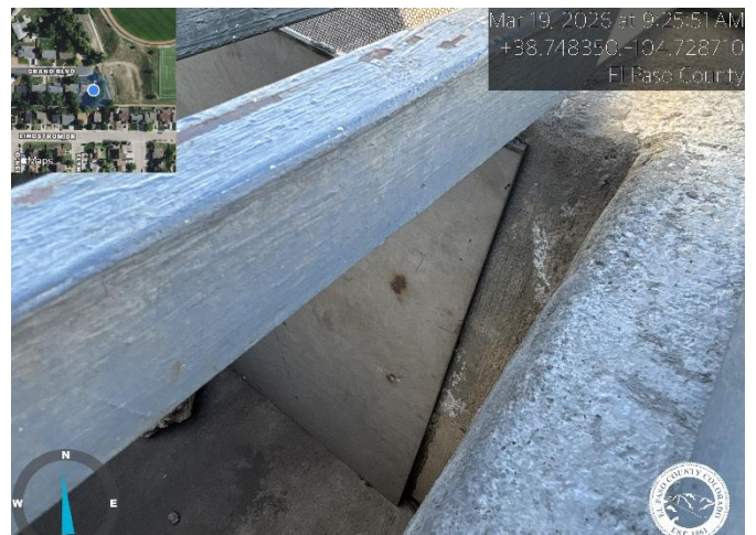
Photo 8: Orifice Plate Gasket is inadequate.
