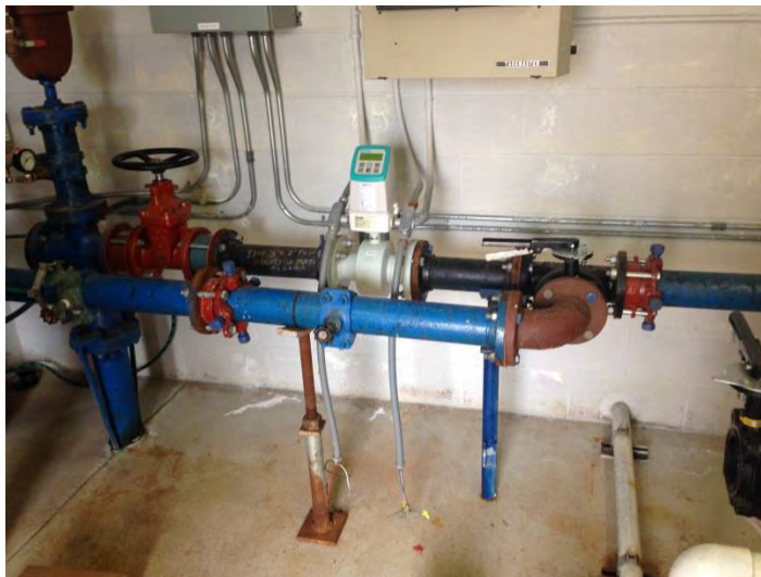
Figure 5: Piping inside Pump House 6
