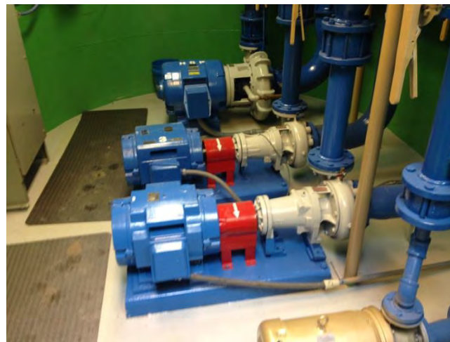
Figure 7: PBHMD Booster Pumps
