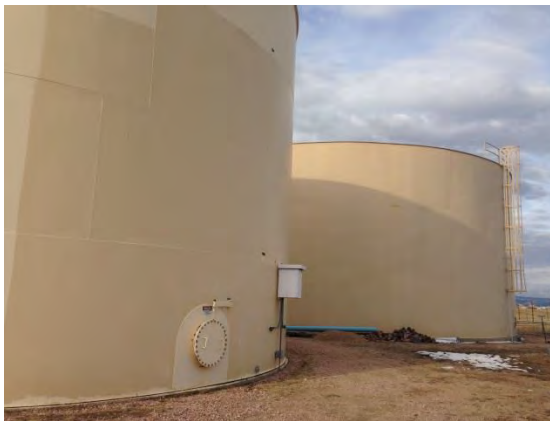
Figure 6: PBHMD 1 MG Water Storage Tank (left) and 0.5 MG Water Storage Tank (Right)
