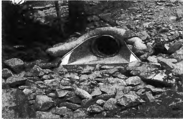
Photograph TOP-1. Riprap outlet protection.
