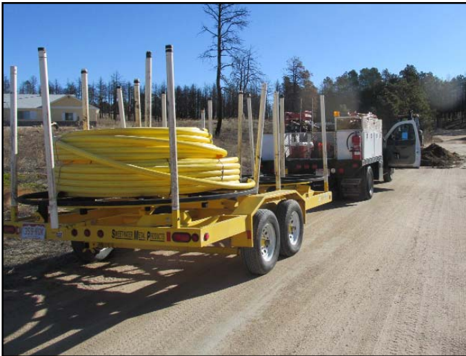
Photos of von Ahlefeldt gas line being installed along north side of Forest Hts Circle in March, 2016. View is top the east. You can see Phyllis' new house (white arrows) in photo above at extreme left center, and also above the backhoe (left) as digging bends to cross the cul de sac. View is to the north.
