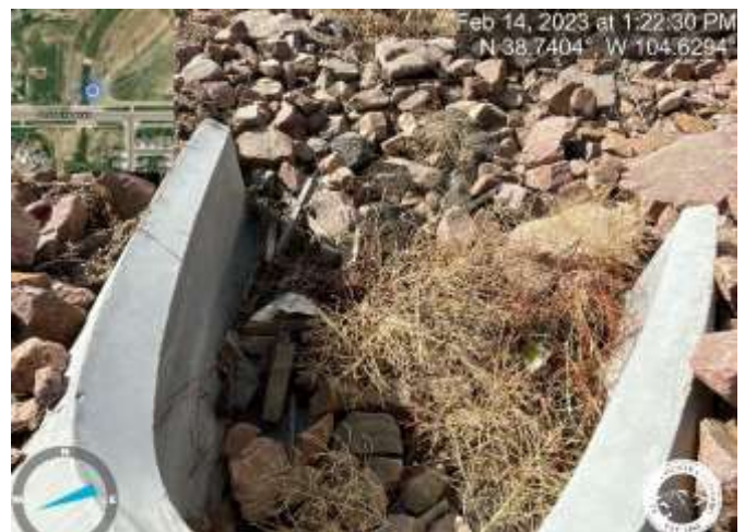
Photo 4: Pond C5: Remove sediment and debris from outlet pipe.
