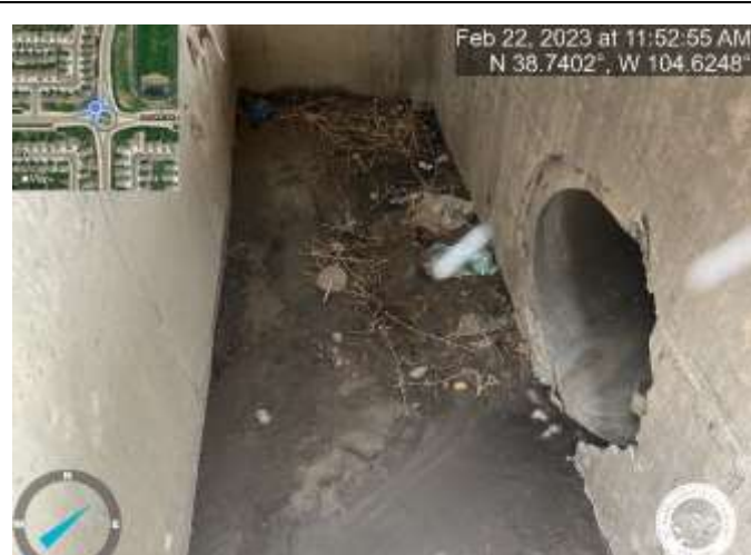
Photo 17: Inlet DP-34: Remove sediment and debris from inlet (inlet is marked with a green dot on the lid).
