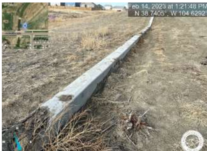
Photo 3: Pond C5: Raise grade to be flush with the Overflow Cutoff Wall.
