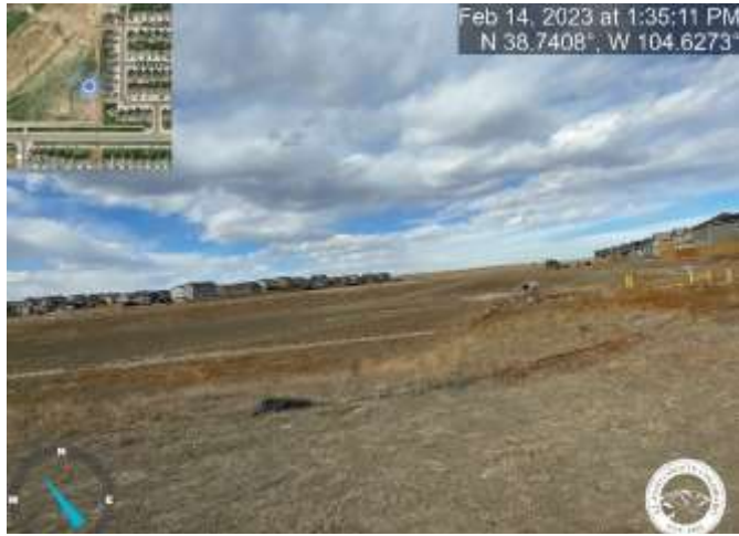
Photo 10: Pond C5: Remove silt fence that was cut to the ground just east of pond C5.
