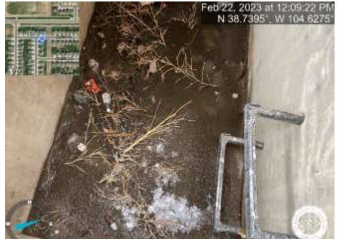
Photo 22: Inlet DP-38: Remove sediment and debris from inlet (inlet is marked with a green dot on the lid).
