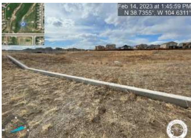
Photo 11: Pond D2: Raise grade to be flush with the Overflow Cutoff Wall.
