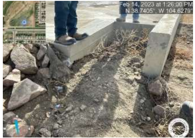
Photo 6: Pond C5: Implement 9" D50 rip rap per specification on forebay B. Reference page C9.2 Lorson Ranch F1 Street, Storm Sewer, and Pond Construction Plans.
