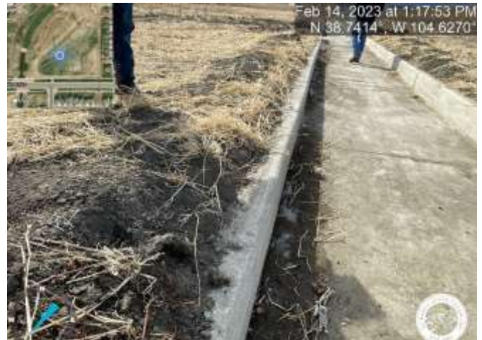
Photo 2: Pond C5: Remove sediment to match the top of trickle channel curb with a 3% slope towards trickle channel for positive drainage.
