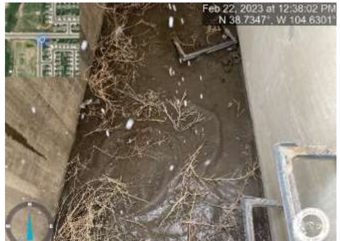
Photo 24: Inlet DP-60: Remove sediment and debris from inlet (inlet is marked with a green dot on the lid).
