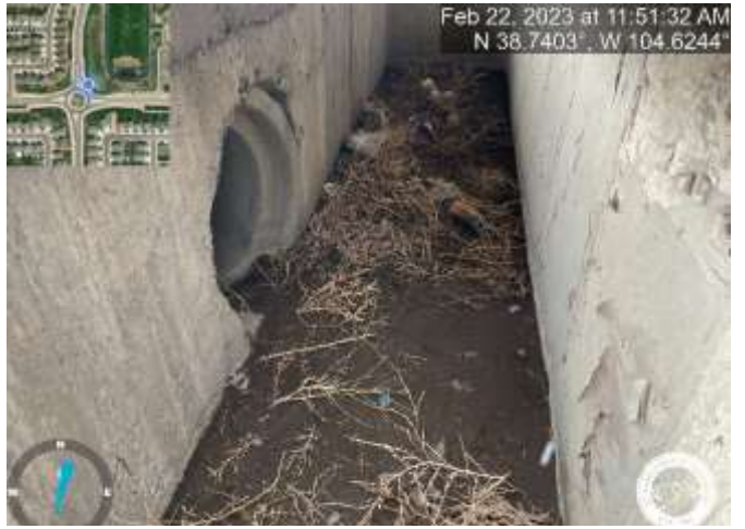
Photo 16: Inlet DP-33: Remove sediment and debris from inlet (inlet is marked with a green dot on the lid).
