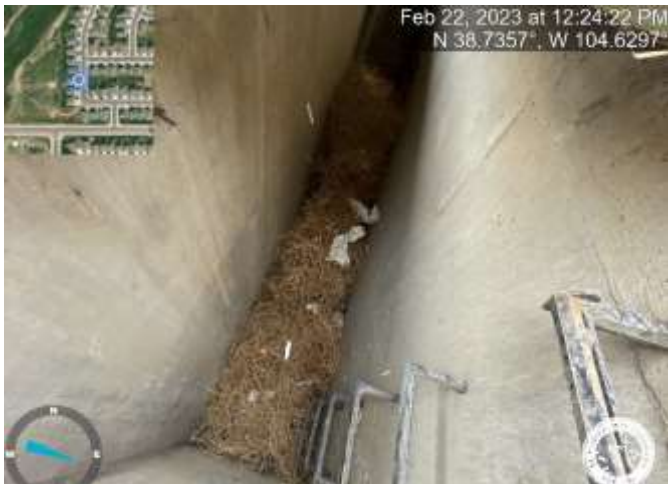
Photo 23: Inlet DP-56: Remove sediment and debris from inlet (inlet is marked with a green dot on the lid).
