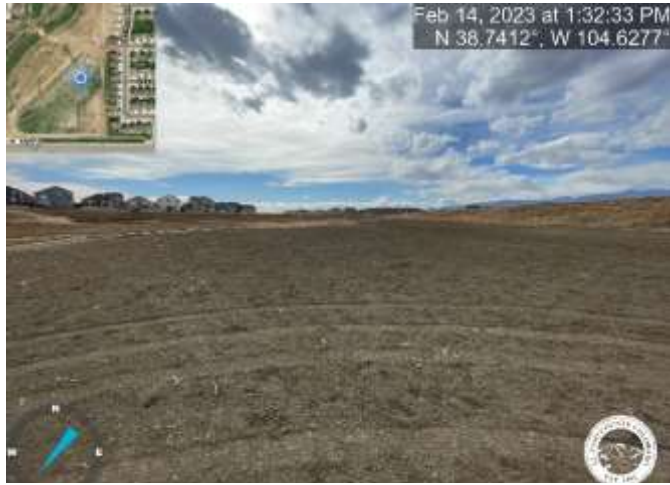
Photo 9: Pond C5: Failure to achieve uniform vegetative cover with an individual plant density of at least 70 percent in pond bottom.
