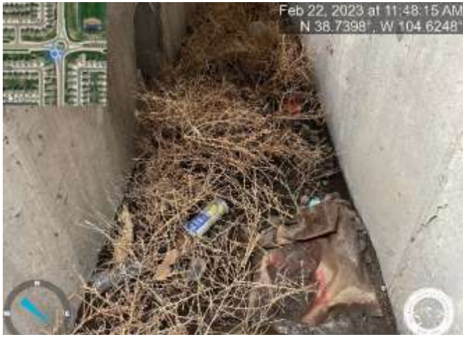
Photo 15: Inlet DP-29: Remove sediment and debris from inlet (inlet is marked with a green dot on the lid).
