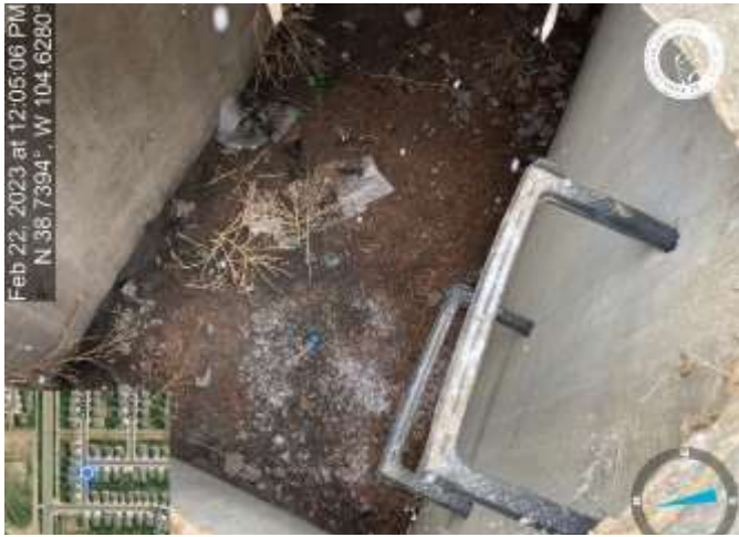
Photo 21: Inlet DP-39: Remove sediment and debris from inlet (inlet is marked with a green dot on the lid).
