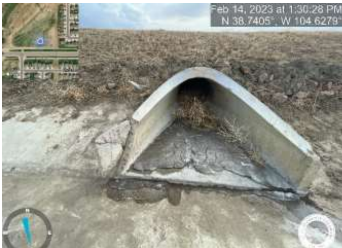
Photo 7: Pond C5: Repair flared end section on inlet pipe to forebay B.
