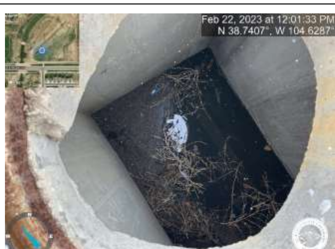
Photo 20: Inlet DP-40: Remove sediment and debris from inlet (inlet is marked with a green dot on the lid).
