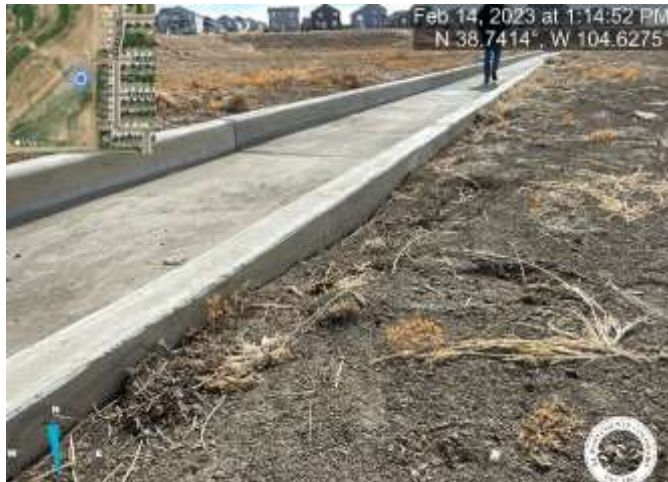
Photo 1: Pond C5: Raise pond bottom to top of trickle channel curb with a 3% slope towards trickle channel for positive drainage.
