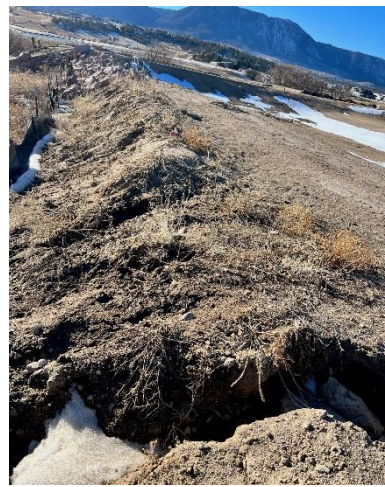
Photo 8. Regrade Pond walls to address erosion along southern perimeter.
