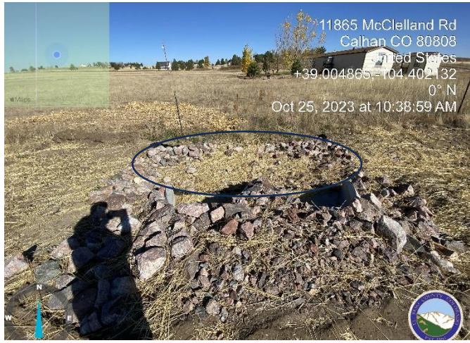
Photo 1: Station eight on road profile, riprap pad on north side not built per plan. Calls for the length to be 10' and the installed product is 8'.
