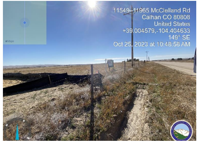
Photo 2: Offsite grading not installed per plan. Grading stops at property line, on plans it shows it extending further.
